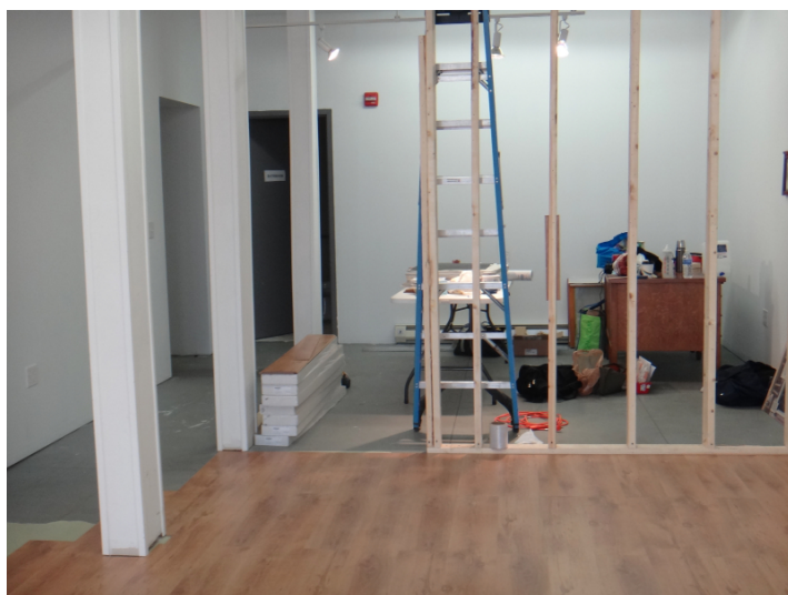
At Cottrill's Opera House in Thomas, the hands-on team laid the floor and put in a wall. Photo by Jenny Hart.
