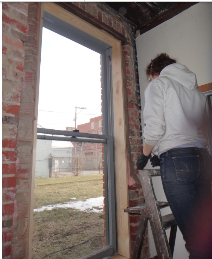
Jenny Hart trimming in windows at the Delmonte. This image shows casing being put in around the windows so trim can be added to the outside. Photo by Kara Baldwin.
