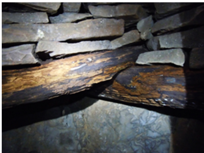
Bedrock, timbers, and stacked rock at the bottom of the well. Taken by Kyle Mills.
